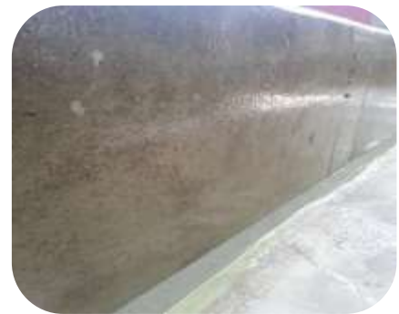
Concrete wall suffering from weather and UV degradation sealed with Resichem 505 Damp Seal
